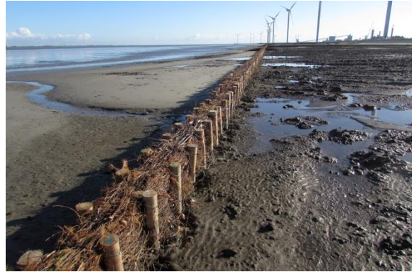
Figure 20 Brushwood groynes at the saltmarshes in Delftzijl (Nature-based salt marsh development in the port of Delftzijl, n.d.).
